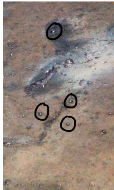
Figure 2. Weld spatters as generated (Highlighted with circles)
